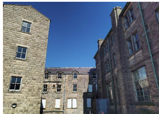
Image 6: Southern roofline. Missing tile at the far eastern edge of the roofline, just above the eastern gable end.
