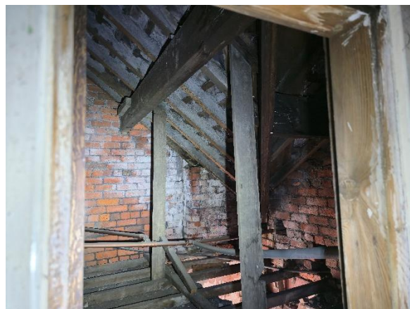
Image 8: Internal view of crawl space and significant deterioration.
