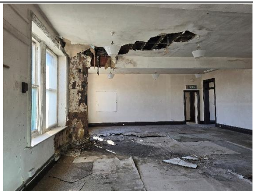
Image 9: An indication of the deterioration within Hardwick Hall.
