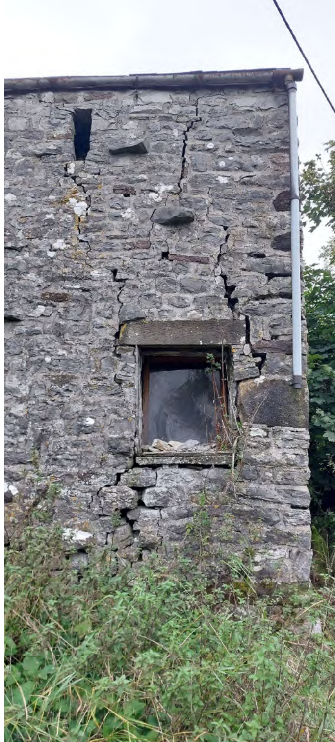
Picture2- Visible vertical cracks and loose stone work in south elevation in the building.
