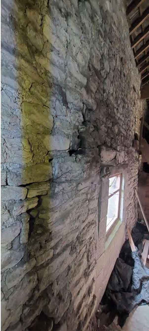
Picture6- The wall misaligned with the perimeter footprint at the central section above lintel.
