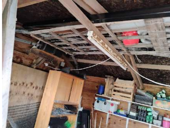
8. Bulky items stored in roof timbers.
