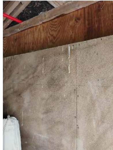
5. Bird droppings on internal partition.
