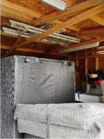
7. Items stored in roof timbers, and bulky stored items in stalls.
