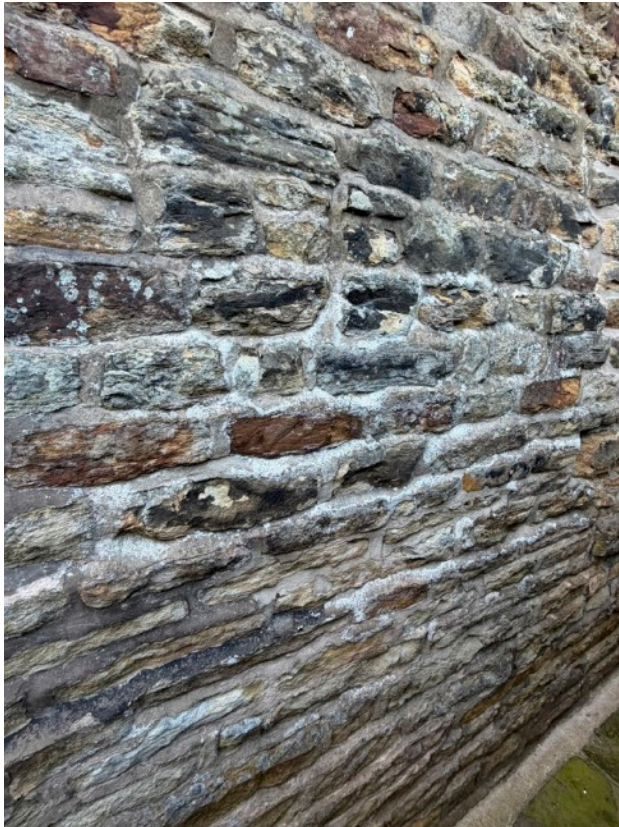
Existing gable wall pointing - Historic poor quality sand and cement repairs which are starting to cause damage to the original stone as they retain moisture and add stains
