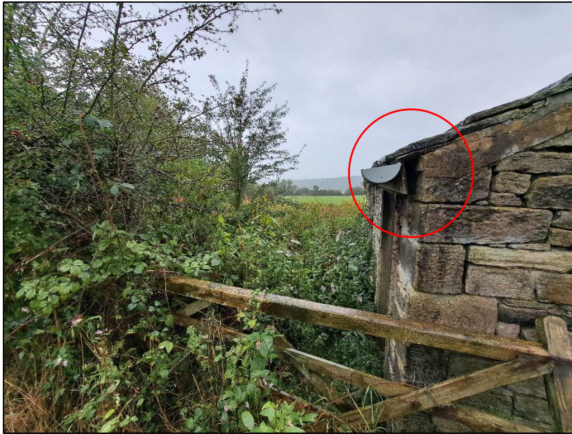
Photograph 4 showing the gap between the roof tiles and soffit
