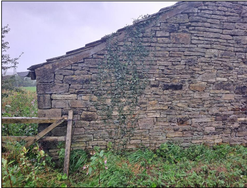
Photograph 2 showing gaps in the external stonework
