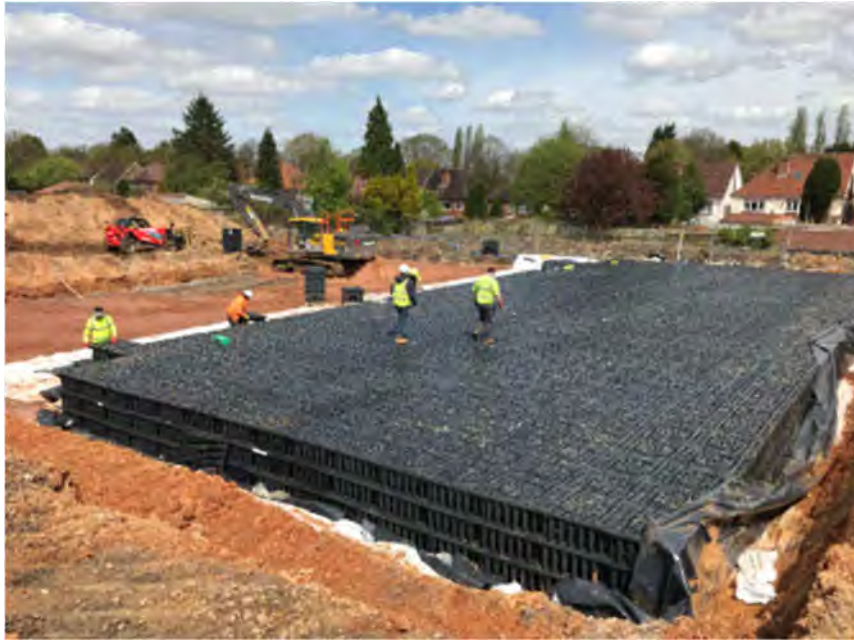
Figures 30. Attenuation Tank.
