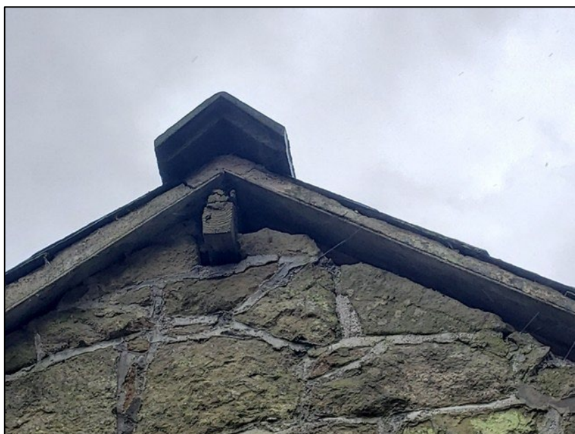
Photograph 6 Showing the roof edge of the single-storey, split-level section on the northern gable of the Coach House with the missing mortar and exposed roof board
