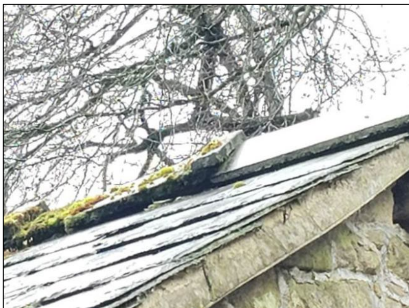
Photograph 8 Showing a lifted ridge tile on the roof of the split-level section on the northern elevation
