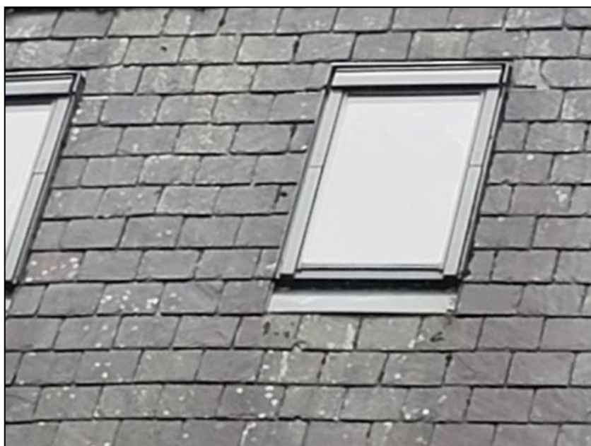
Photograph 9 Showing an area at the base of the skylight on the main roof, which is lifted away from the roof tiles
