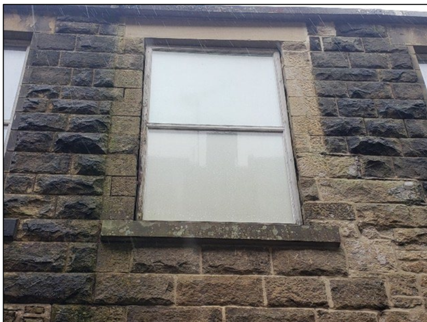
Photograph 4 Showing evidence of more recent works to first-floor windows, with surrounding small gaps and the associated newer masonry
