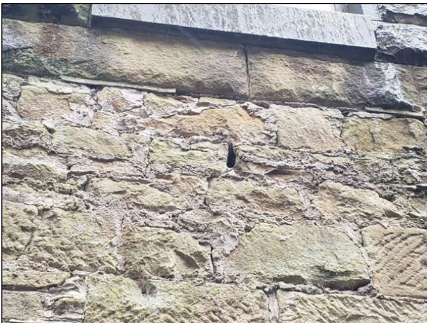
Photograph 2 A section of missing mortar within the southern elevation stonework
