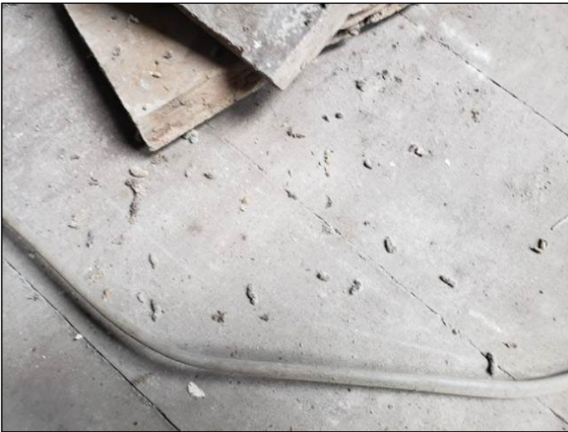
Photograph 19 Showing the accumulation of bat droppings within the western gable void, with a covering of dust
