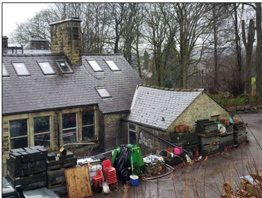
Photograph 7 Showing the northern elevation roof with some missing or cracked tiles visible on the (smaller) split-level section
