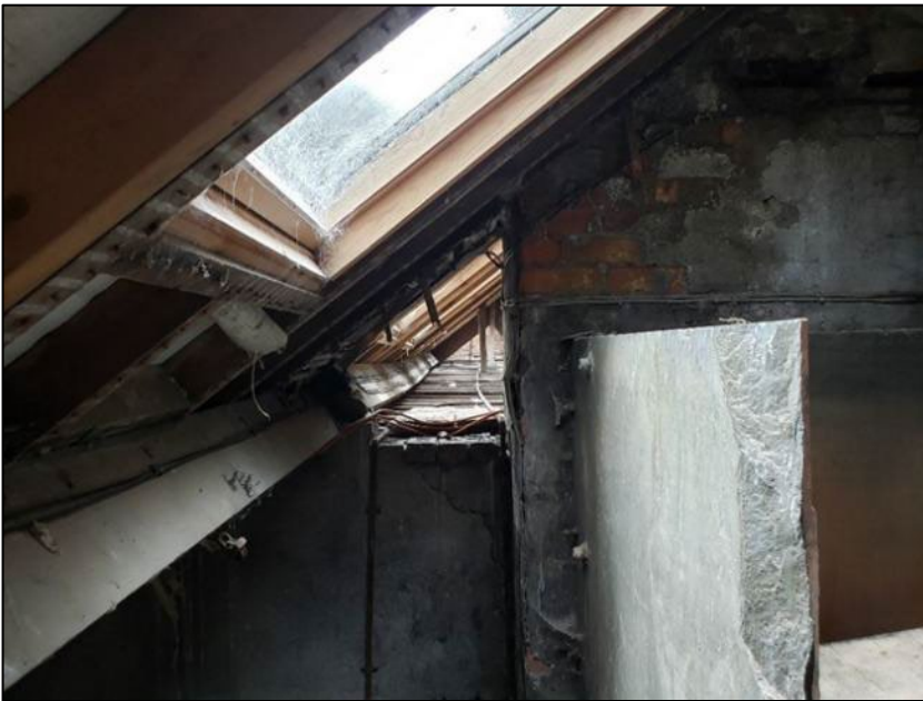
Photograph 16 Showing the void above the western gable rooms which is open to the remaining first floor
