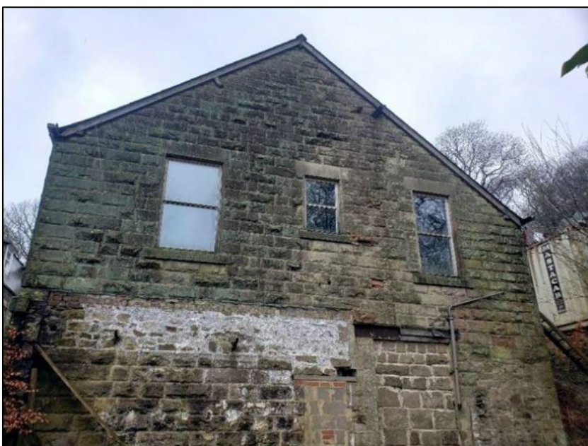
Photograph 3 Showing the evidence of a previous extension on the eastern elevation and the associated gaps along with gaps and crevices at the gable behind the bargeboard
