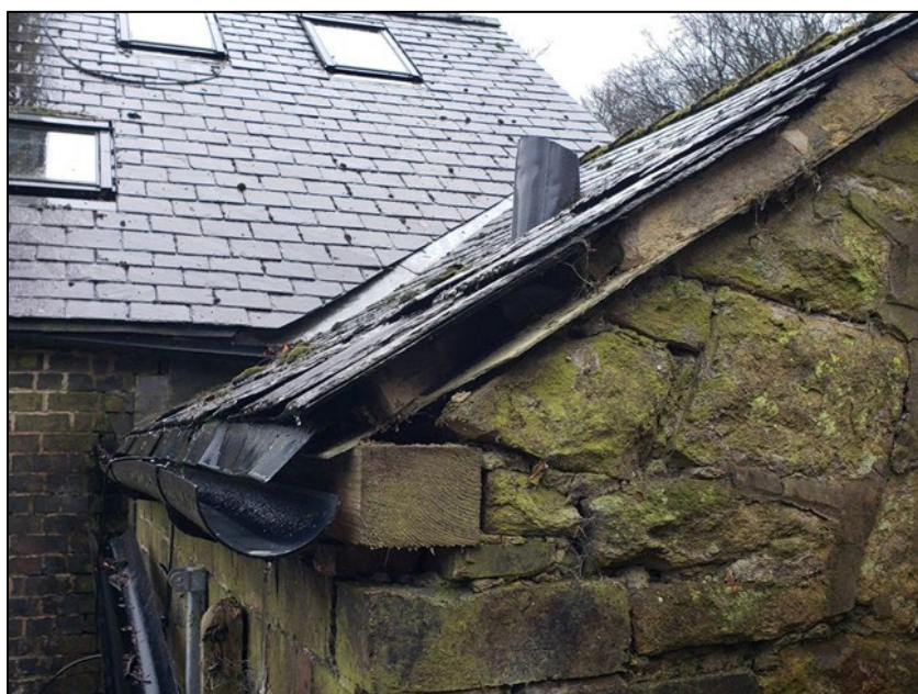
Photograph 5 Small split-level section on the northern elevation which shows an example of the condition of the roof edges at the gables of the building
