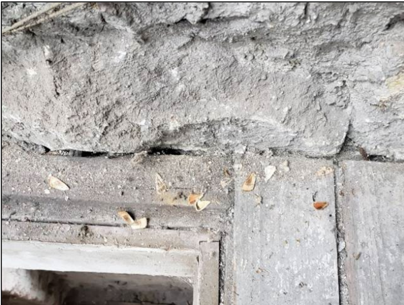
Photograph 14 Showing the accumulation of feeding remains within the eastern gable void, likely from a yellow underwing moth species
