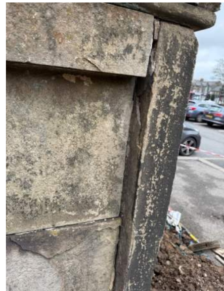
Photo 6 – Severe displacement to south-east corner of cistern; past cementitious repairs noted
