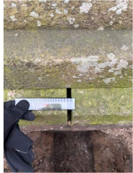
Photo 4 – Separation of plinth stone
