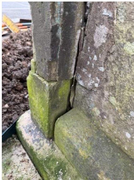
Photo 5 – Severe displacement and fracturing to north-east corner of cistern; past cementitious repairs noted
