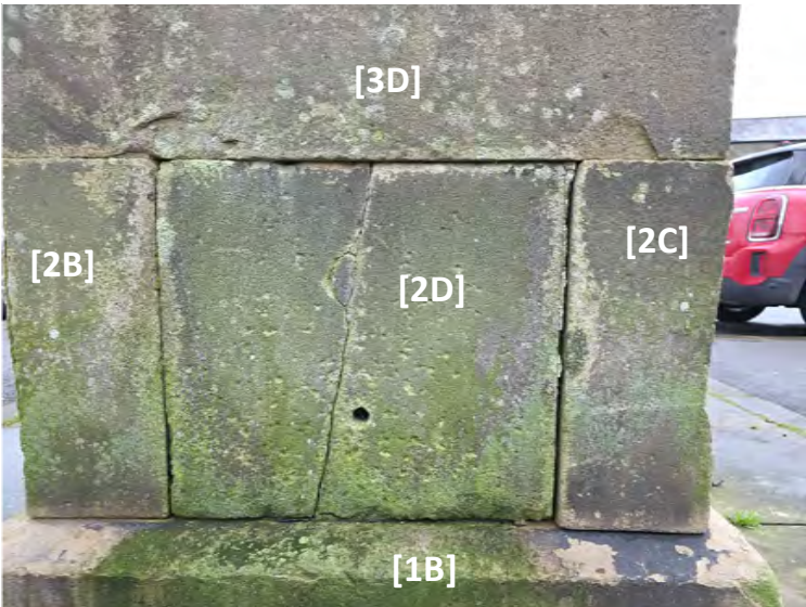
Severe cracking >10mm (Type B defect) through full depth of lower Cenotaph west facade central panel [2D] with minor surface delaminating including impact damage less than 8mm. (Type C.3 Defect) across lower section of panel.
