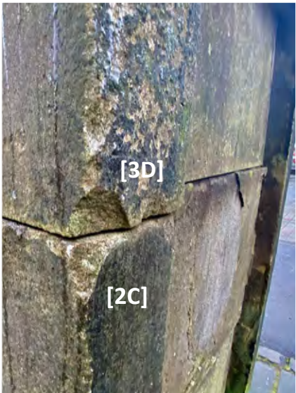
Severe surface deterioration >10mm spalling (Type C1 defect) between panels [2C] and [3D] on southwest corner.
