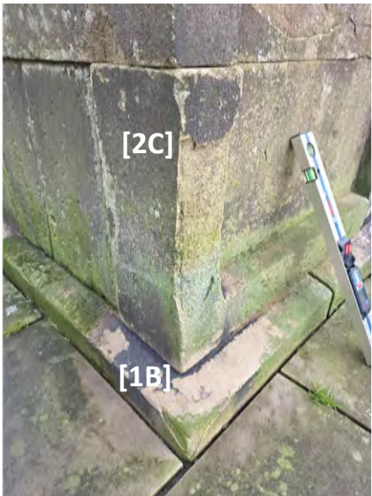
Severe surface deterioration >10mm spalling (Type C1 defect) to southwest lower corner of Cenotaph panel [2C].
