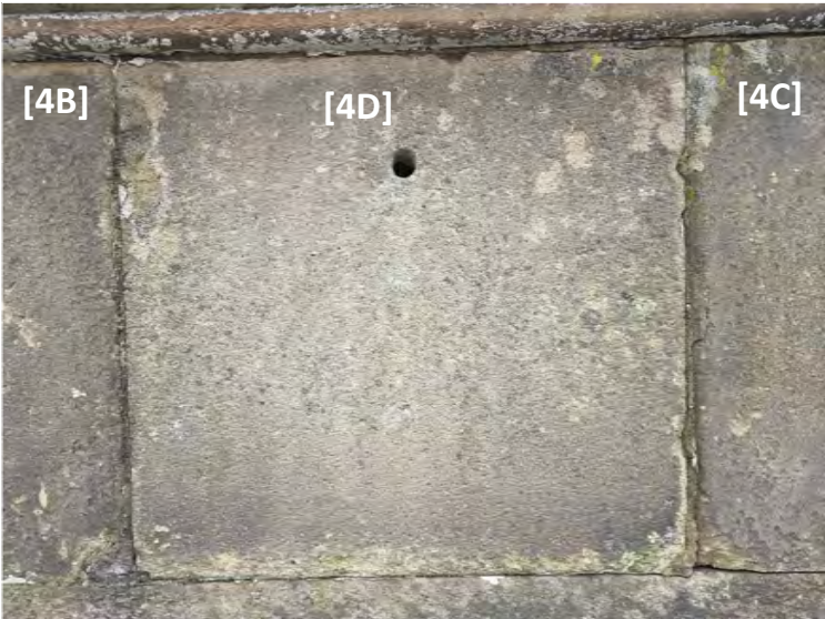
Portland Cement perp end mortar pointing (D1 Defect) to fill structural displacement gaps <10mm and loss of surface to upper panels [D4], [C4] and [B4] of Cenotaph west elevation.
