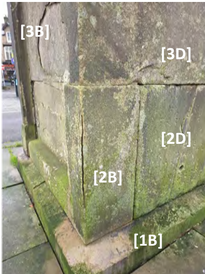
Ashlar in process of delamination - exhibiting bulging (C4 defect) and severe full depth cracking (Type B Defect) [2B] resulting in imminent loss of ashlar fabric.
