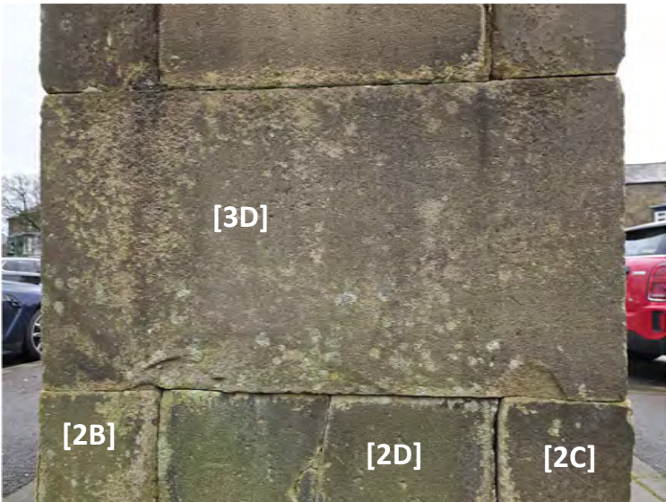
Surface deterioration spalling >10mm (Type C1 defects) to lower section of Cenotaph west elevation mid panel [3D] resulting in loss of ashlar fabric.
