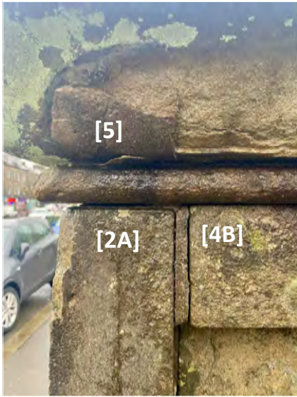
Portland cement pointing between [4B] and Cavindish Motif frame [2A] incl. loss of corner surface to latter.
