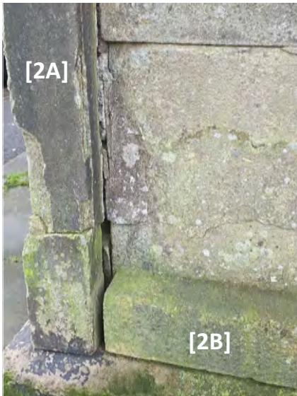
Severe cracking (Type B defect) at the lower northeast corner of the Cavendish frame [2A] with displacement opening up gap to lower north elevation panel [2B] incl. loss of fabric.
