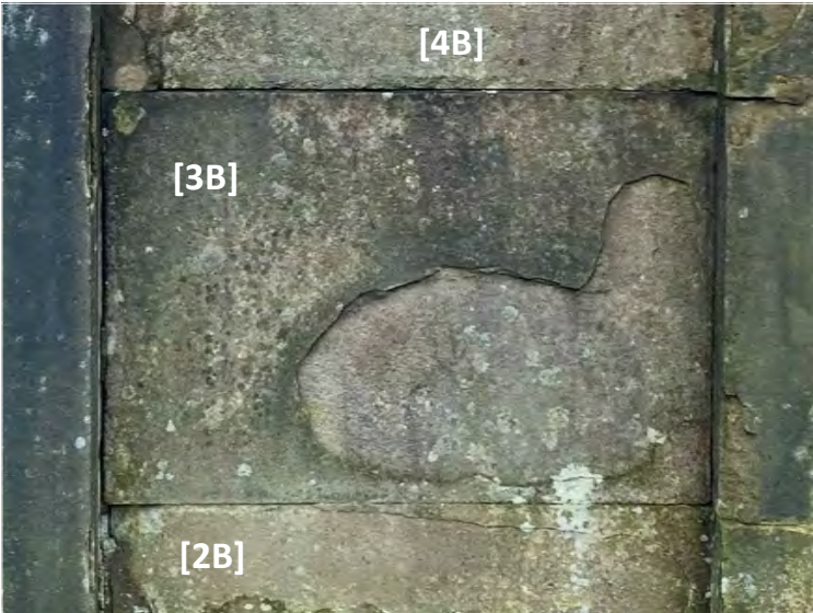
Surface deterioration spalling >10mm (Type C1 defects) Cenotaph north elevation lower panel [B3] resulting in loss of ashlar fabric.
