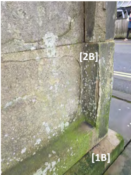
Surface loss to lower panel [2B] and blown surface to NW corner above Plinth [1B]
