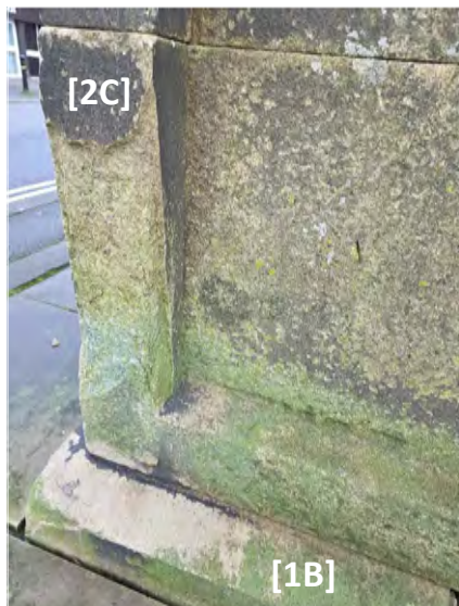
Southwest Corner severe surface deterioration >10mm spalling (Type C1 defect) to southwest lower corner of Cenotaph panel [2C]
