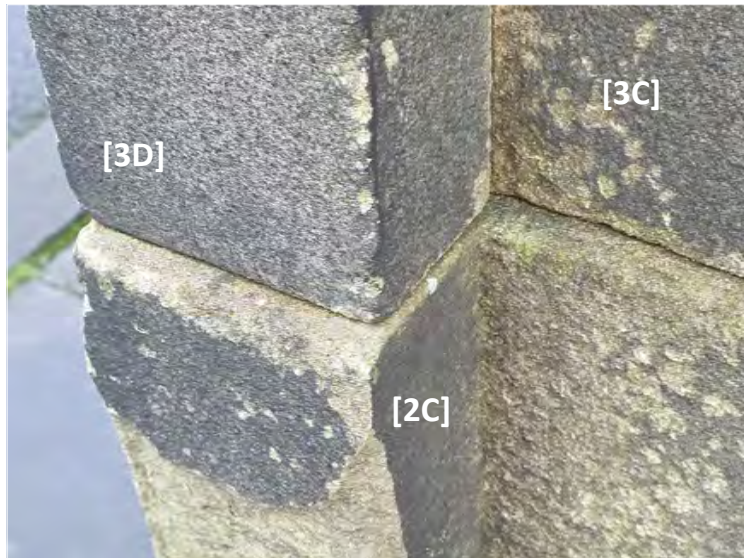
Example of structural displacement (Type A defect) with lower panel 2C pushing southwards below panel [3D]
