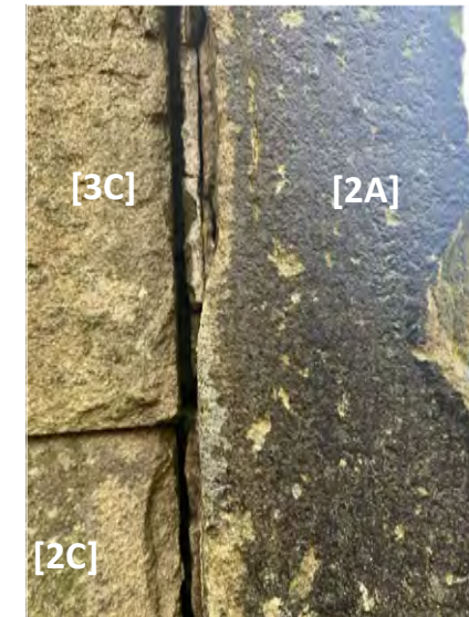
Portland Cement (D1 Defect) to fill structural displacement gaps >10mm between panels [2C], [3C] and [2A].
