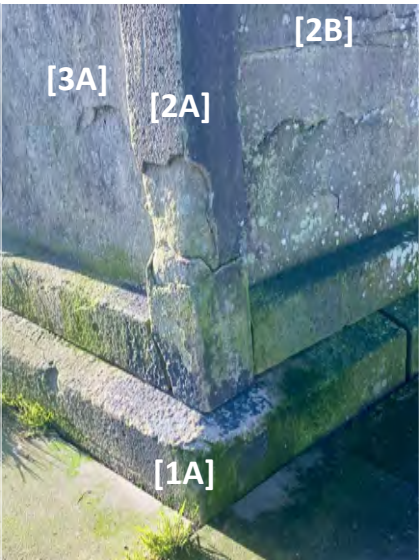
Extent and depth of surface loss to lower NE corner of Cenotaph frame [2A]
