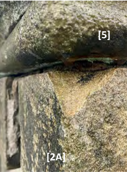
Loss of surface at top southeast corner of panel [2A]
