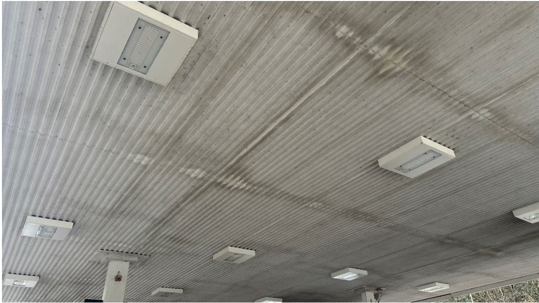
Photo 10: No joints or gaps present throughout the canopy cover.
