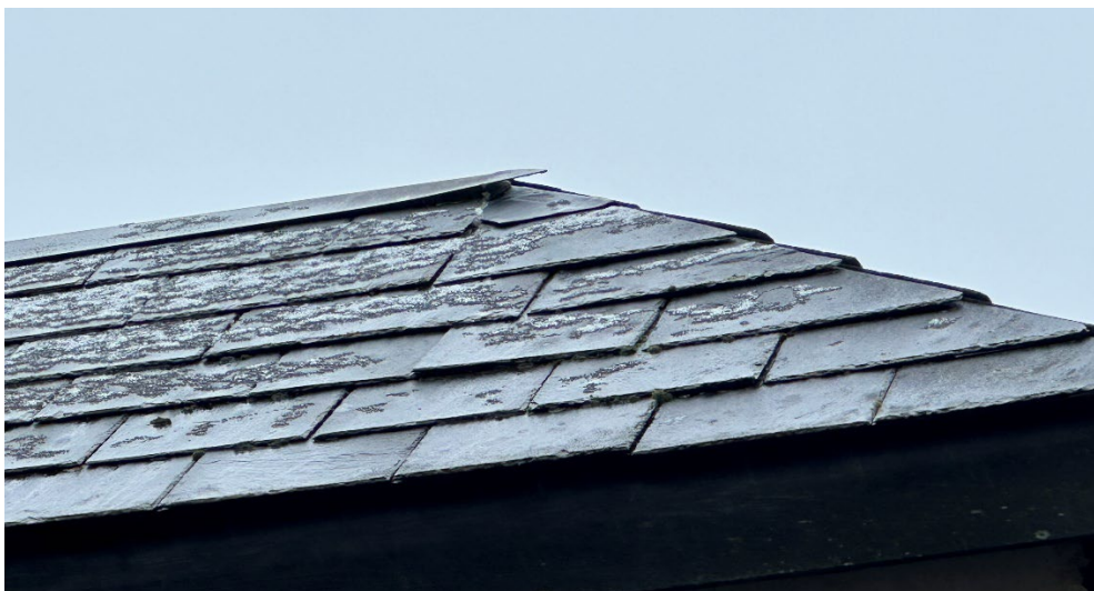
Photo 3: The capping at the top of the ridge is lifted in areas providing PRFs.
