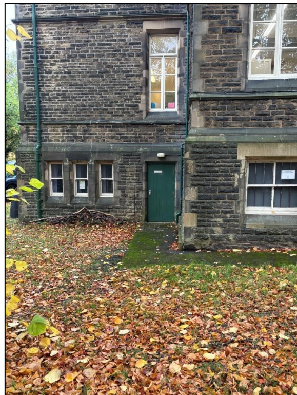
Image 02 Degraded footpath and trip hazards to access
