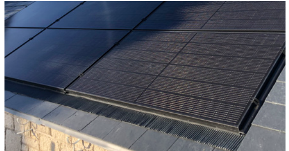
In-roof solar PV panels
