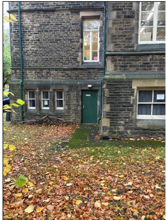
Image 02 Degraded footpath and trip hazards to access
