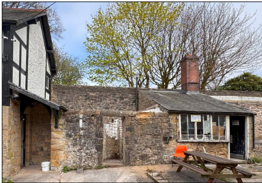
Figure 3: Southeast elevation of the Gardener's cottage showing the dilapidated Toilets and Garden Room
