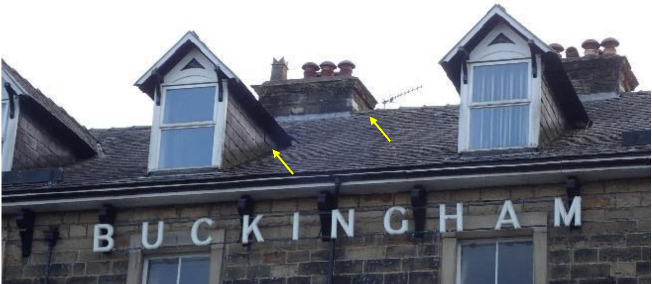
Photograph 5: West aspect of Buckingham Hotel with gaps noted underneath raised slates
