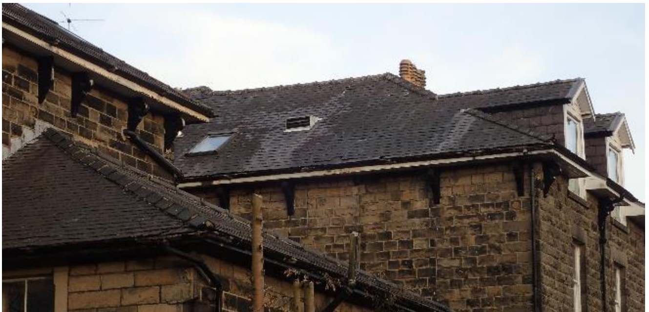
Photograph 4: Roofs at west aspect and rear of Buckingham Hotel where numerous gaps were identified beneath the ridge tiles
