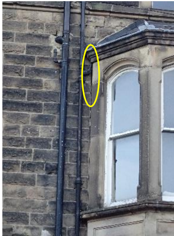
Photograph 6: East elevation of Buckingham Hotel with gap indicated in stonework adjacent to bay window
