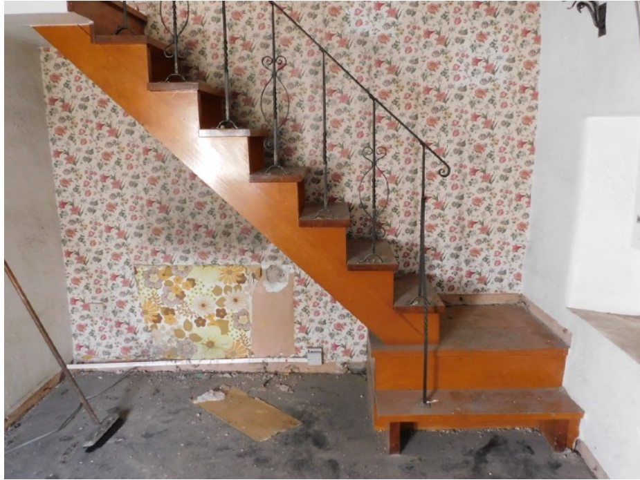
Internal timber staircase - not original and does not comply with building regulations
