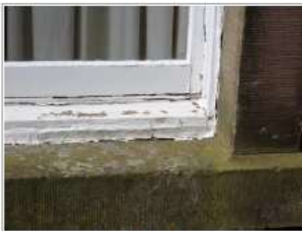
Rotting timber frame
