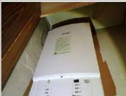
Gas fired boiler
