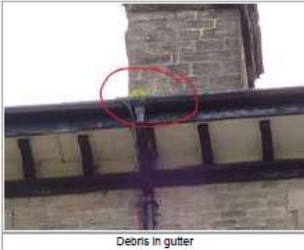
Debris in gutter
