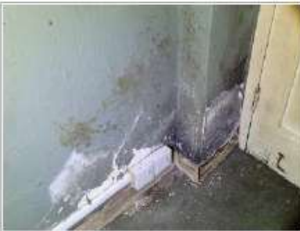
Mould and damp
