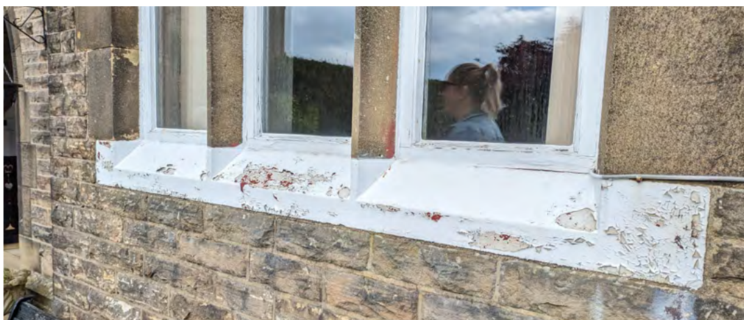
Figure 4 Example of paintwork peeling to external stone surround to lounge window.
