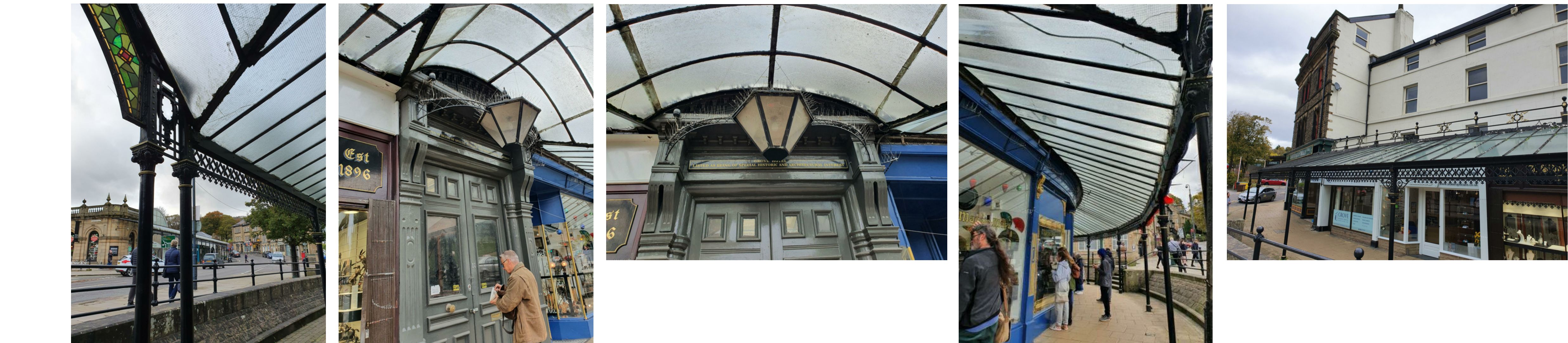
1. View: US of glass canopy over main entrance indicating broken panels to be replaced. 2. View: US of glass canopy over main entrance indicating broken panels and debris over main entrance door. 3. View: US of glass canopy over main entrance indicating broken panels and debris over main entrance door. 4. View: US of glass canopy looking towards retail unit (Maggie Mays) indicating broken panels - to be replaced 5. View: Top of glass canopy looking towards retail unit (Lavender Green) indicating existing condition of paintwork - paint work to be made good (colours to match existing)
