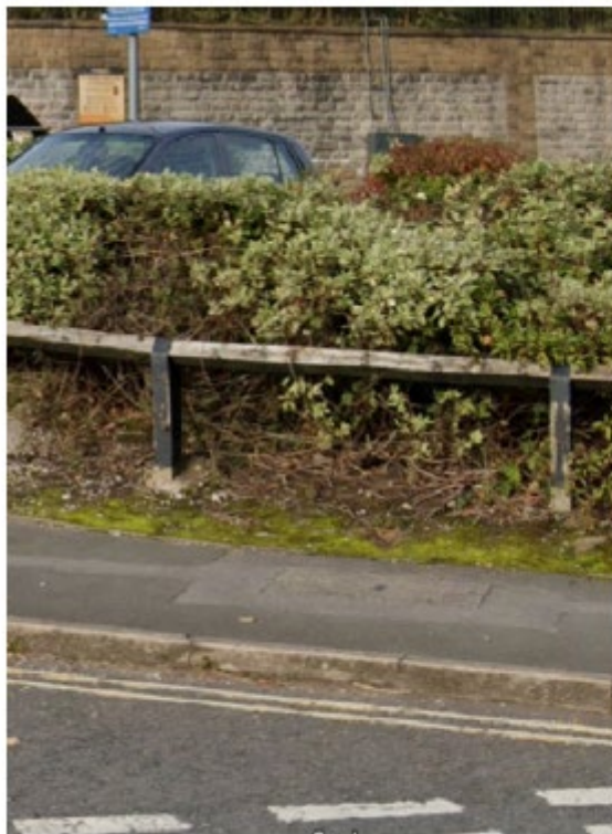
7. Existing timber knee rails in poor condition - To be removed
