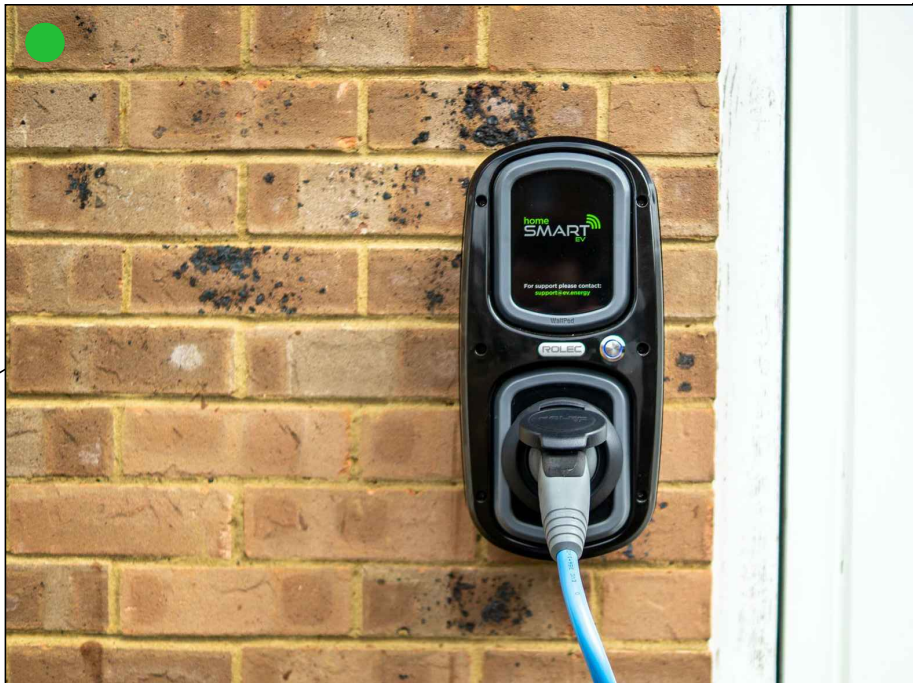
Example of wall mounted EV charging point - Mode 3.
