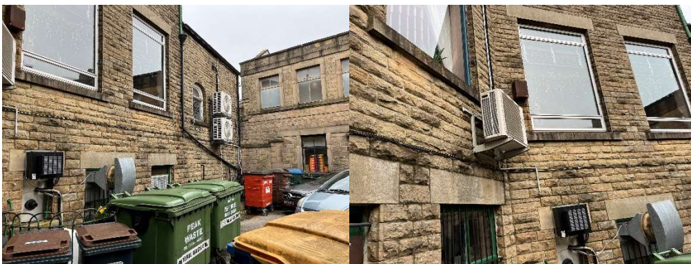
External Plant locate at the rear Associated with other Businesses
