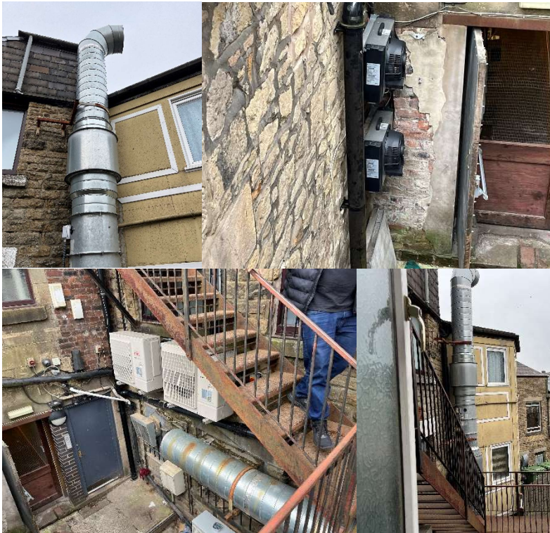
Figure 5 – External plant associated with other businesses
