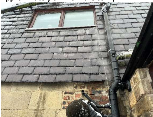
Figure 4 – Nearest Receptor (windows at Approximately 6m from the cowl)
