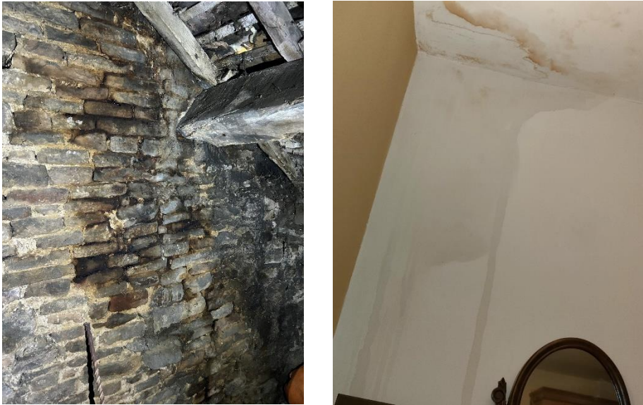
Internal Images of Water Ingress
