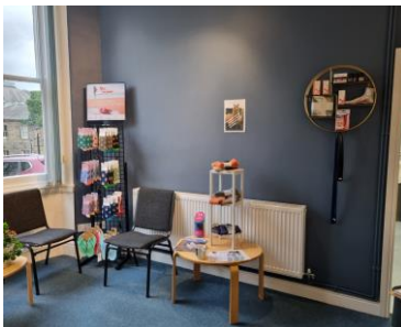
Figure 4: New radiator R2
