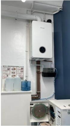
Figure 2: New boiler to Clean Room external wall, gas engineer has confirmed that this has been fixed to the wall using wallplugs installed in the external wall to a depth to ensure that the wall is not compromised structurally or in terms of moisture ingress. Also visible is the flue from the boiler.
