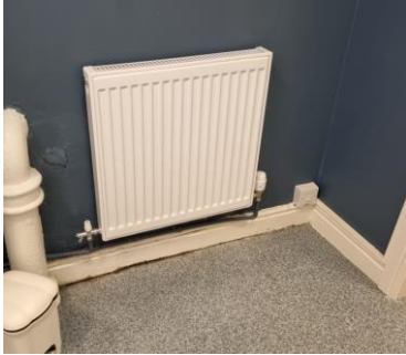
Figure 8: New radiator R6
