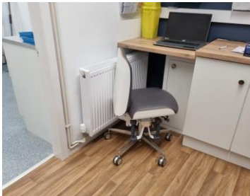
Figure 6: New radiator R4
