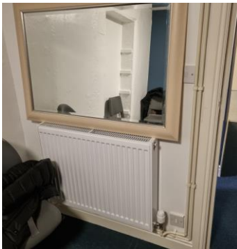
Figure 7: New radiator R5
