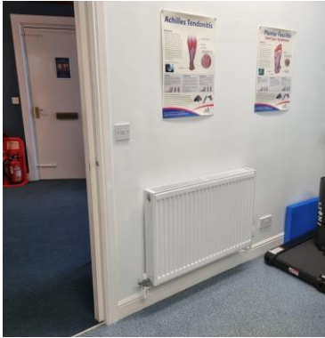
Figure 3: New radiator R1
