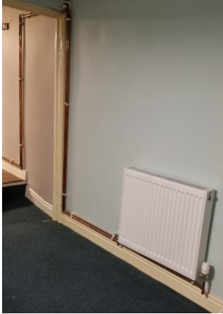
Figure 10: New radiator R8
