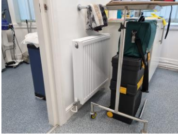
Figure 5: New radiator R3
