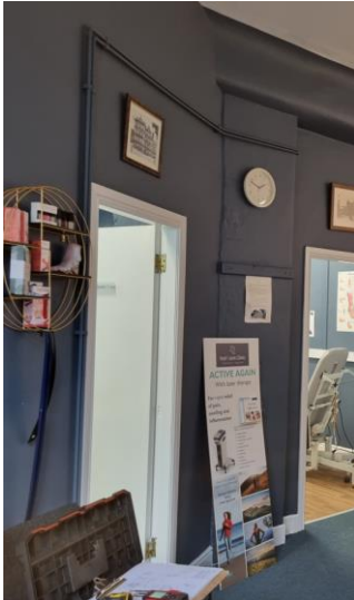
Figure 11: Surface fixed central heating pipework to Reception area noting the small pipe fixings to the wall.
