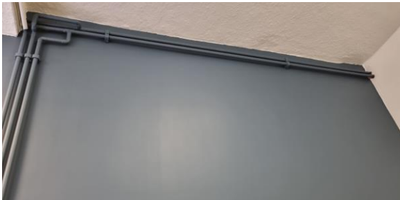
Figure 12: Surface fixed central heating pipework to the UA WC noting the small pipe fixings to the wall on the vertical and horizontal installations.
