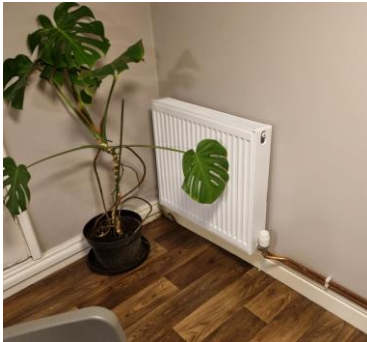
Figure 9: New radiator R7
