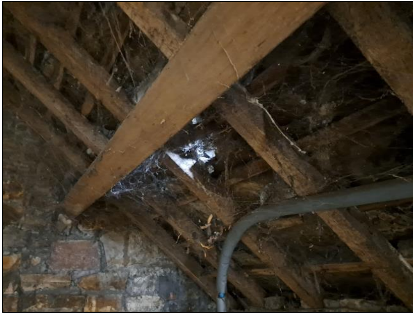
Photograph 9 showing a gap in the tiles
