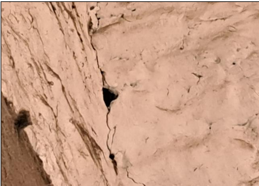
Photograph 12 showing a gap in the wall
