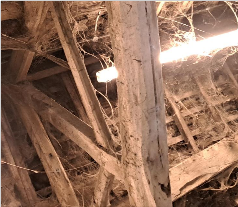
Photograph 11 showing gaps in the timber
