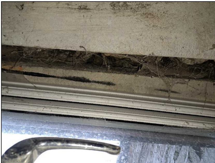
Photograph 10 showing a gap in the lintel
