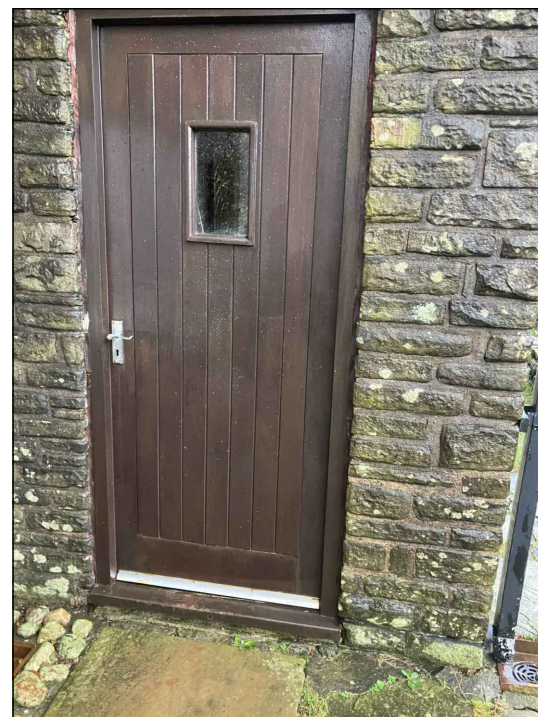
4.Detail photograph of existing stained HW front door and surround. Door and frame to be replaced
