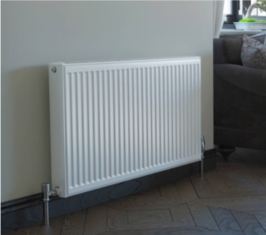
Stelrad Compact Radiator located in the lounge and bedroom
