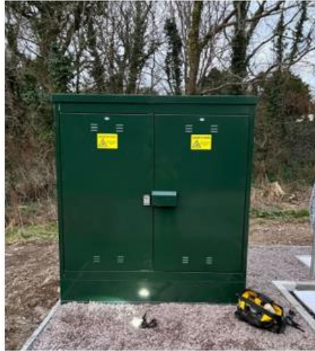
Figure 3: Feeder Pillar RMC 2100
