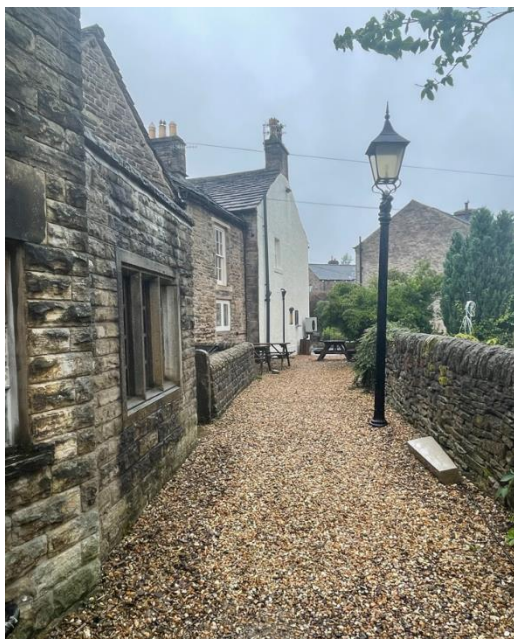
Figure 4: View of northern elevation from east approach. Historic building elements to the east, more modern fenestration and Finish to the west end of the northern elevation. The small opening sits to the west end of the northern elevation. Due to its size and location within the later addition its visual impact upon the heritage asset is low.
