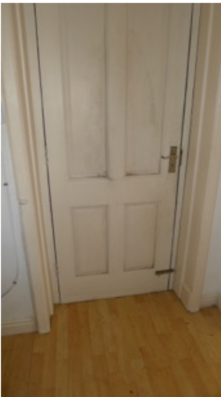
Poor condition to external rear kitchen doors
