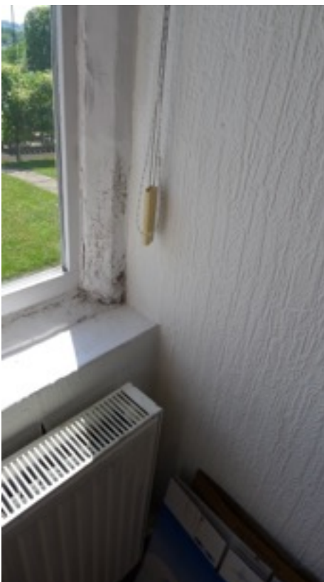
Condensation build up to mullioned bay window
