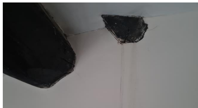
Fig.7 Evidence of Internal leaking occurring within upper bedroom space
