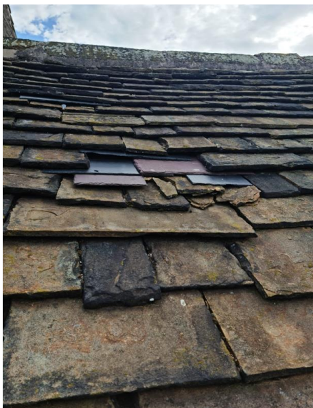
Fig.6 existing roof covering to rear elevation – inadequate temporary repairs been carried out previously.
