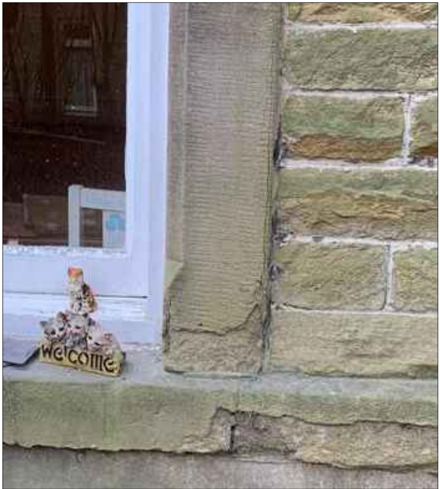
EXISTING PLINTH SHOWING SIGNS OF AGEING
