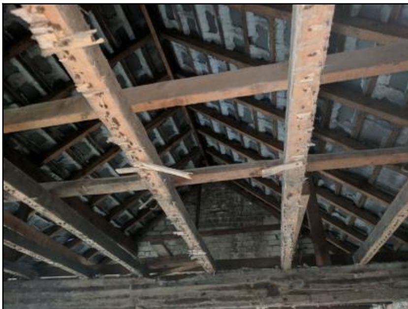
Photograph 7 showing the upper floors with removed ceilings
