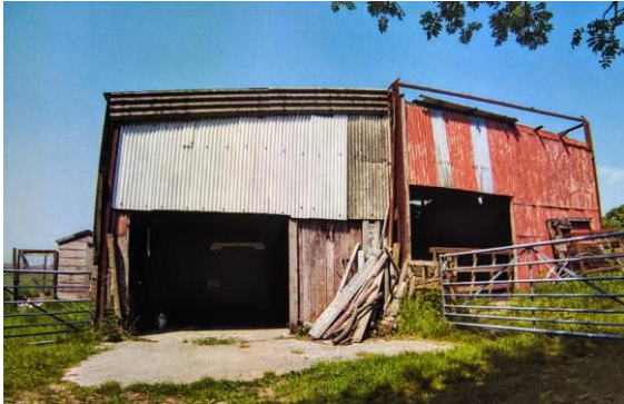
Figure 3: The original Agricultural Building on the footprint prior to deterioration.
