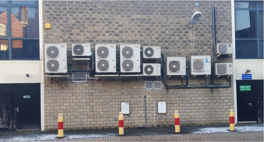
Figure 6 – Wall mounted condensers on opposite wall of retail units
