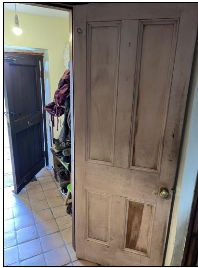
Figure 11: D2 internal door.
