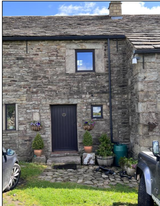
Figure 11: The existing masonry on the affected areas of the southwest and northwest walls.
