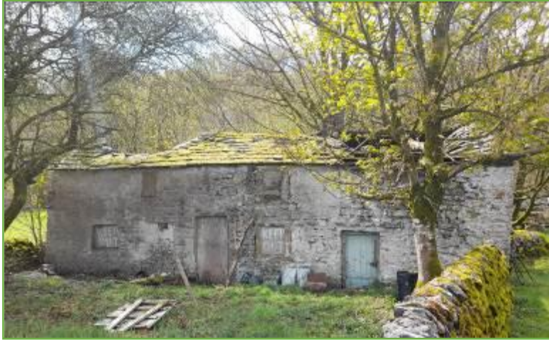
Picture 1: Front view showing extent of damage
