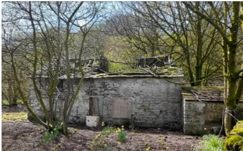
Picture 2: showing surrounding tree cover and roof damage
