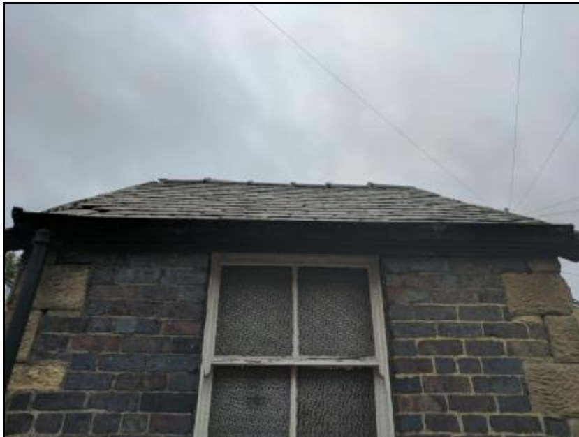
Photograph 5 showing the exterior of the small storage building attached to the rear extension
