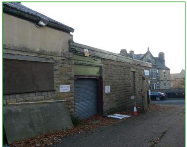
The north elevation of Building 1 showing part of the flat-roof stone section and the brick, pitched-roof section
