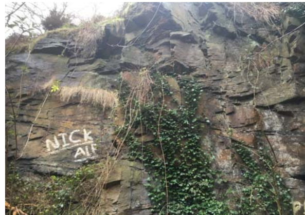
Photograph 2 Rock Face exposure in the Southeast corner of the site showing massive gritstone overlain by thinner beds above (overhanging).
