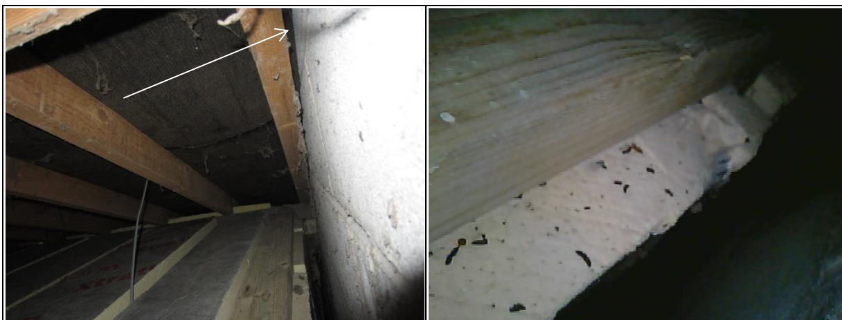
Photograph 7: View of southern gable wall. Roost site between rafter and wall – note bat dropping adhered to wall
