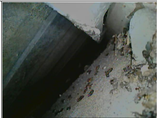
Photograph 4: Bat droppings between felt and roof tiles
