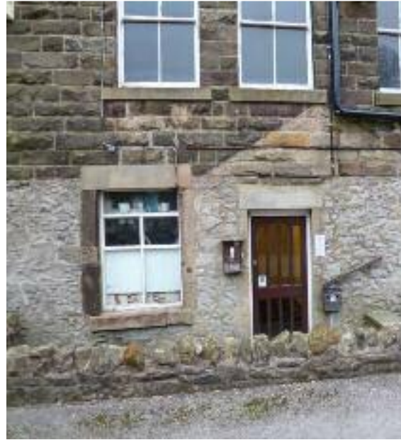
Rear elevation with random limestone to basement level and scarring from a removed addition.
