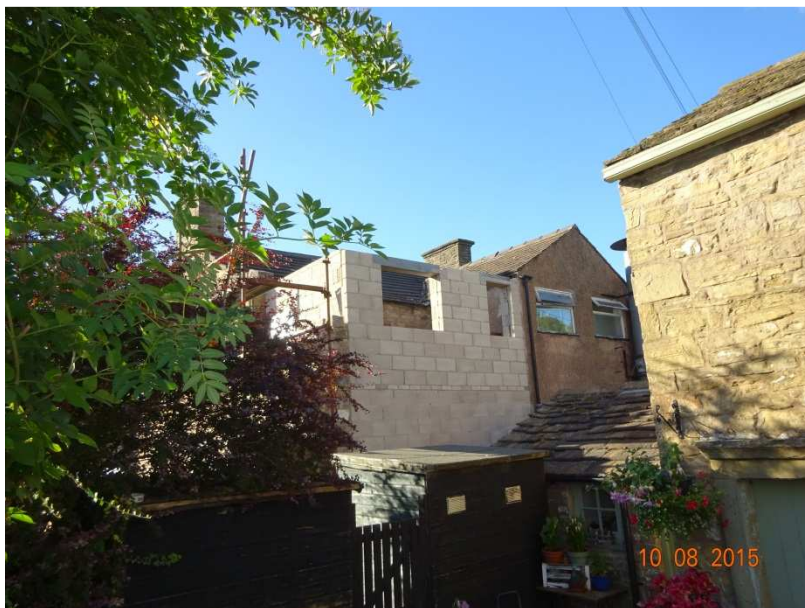
Photo showing rear of 110 Buxton Road with part of proposed extension constructed
