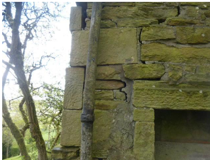
Figure 6 - cracking to left hand side of door reveal
