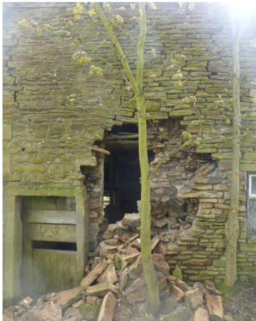
Figure 5 - central collapsed area
