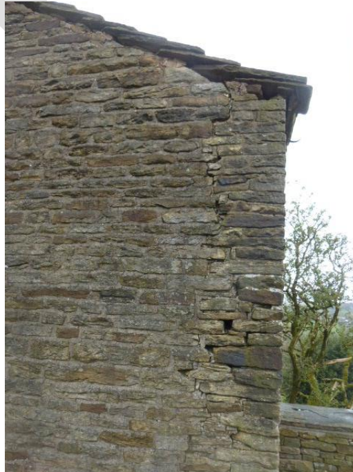
Figure 8 - cracking to rear corner arris
