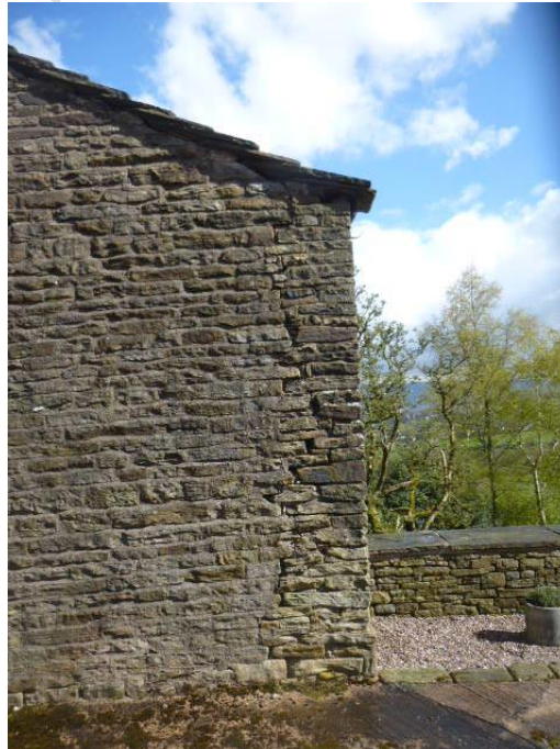
Figure 3 - cracking to arris
