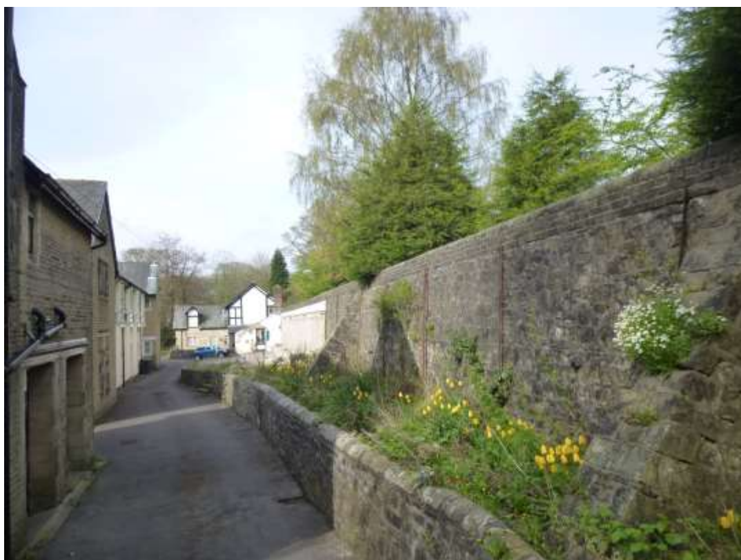
P6: View south west along rear boundary wall.
