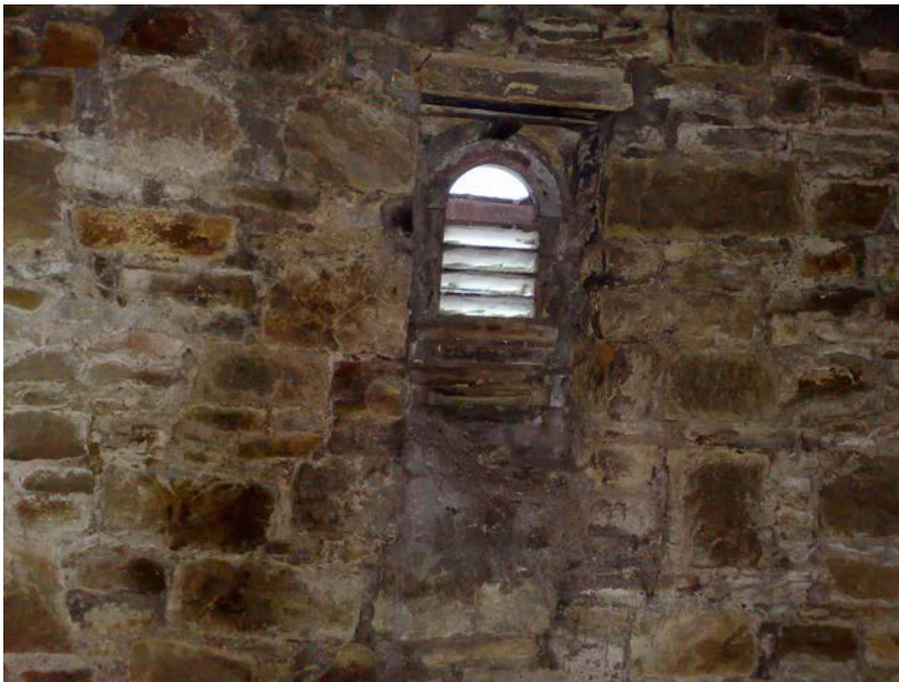
Figure 10. Main roost access point in west end of Brookbottom Methodist Church. Note cavity above window frame.
