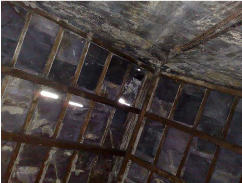
Figure 11. Vestry roof showing spaces between tiles in Brookbottom Methodist Church.
