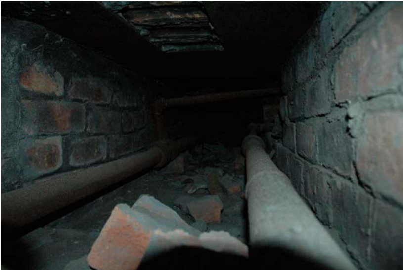
Figure 8. Cavities in cellar at Brookbottom Methodist Church.
