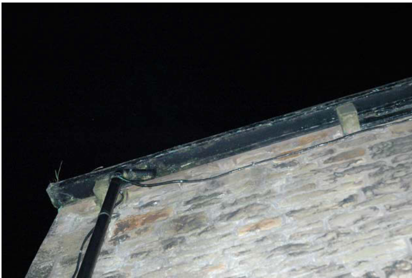
Figure 14. Missing fascia board on western end of south wall, showing roost entry point.
