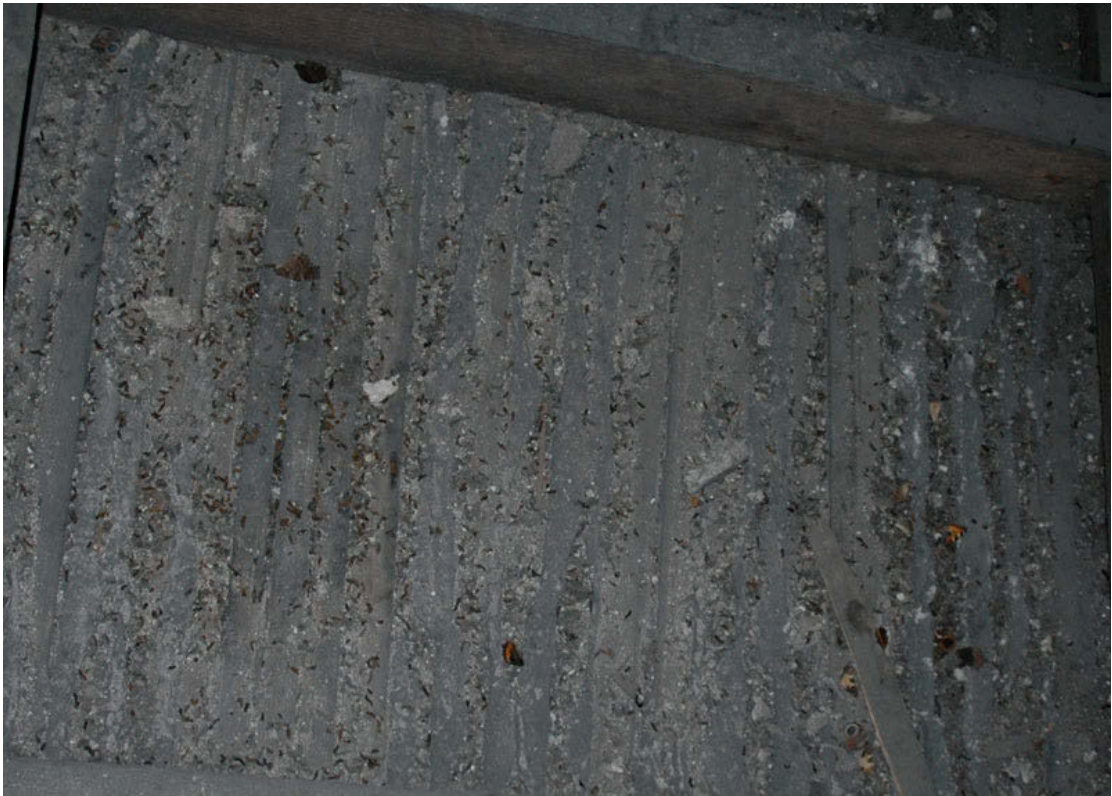
Figure 16. Faeces/feeding signs of bats in the church attic.
