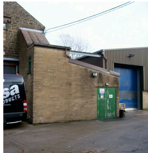
Fig.4 Building M3- Access Stairwell. Demolish to provide maneuverability on within the yard.
