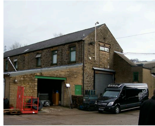
Fig.3 Building M2- Lean to near side of Bowden Hey Road. Demolish due to structural stability which has deemed it unusable.
