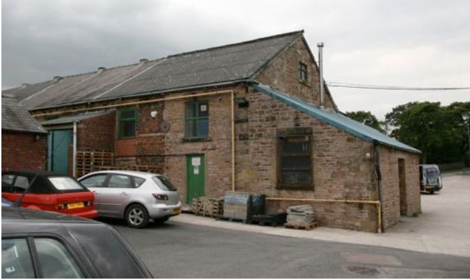
Fig.2 Building M1- Extension to the South West Mill. Demolish to provide maneuverability on site and to create boundary between what will be Residential & Industrial.
